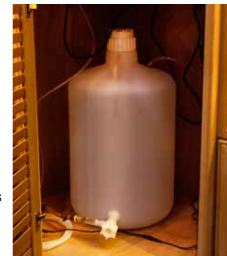
Water Tank Reservoir
